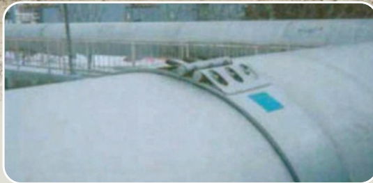
▲ 48" (1,200A) MF-RL Canadian power plant cooling line
