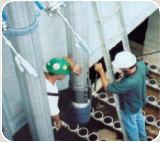
▲ Canada: water purification facility
