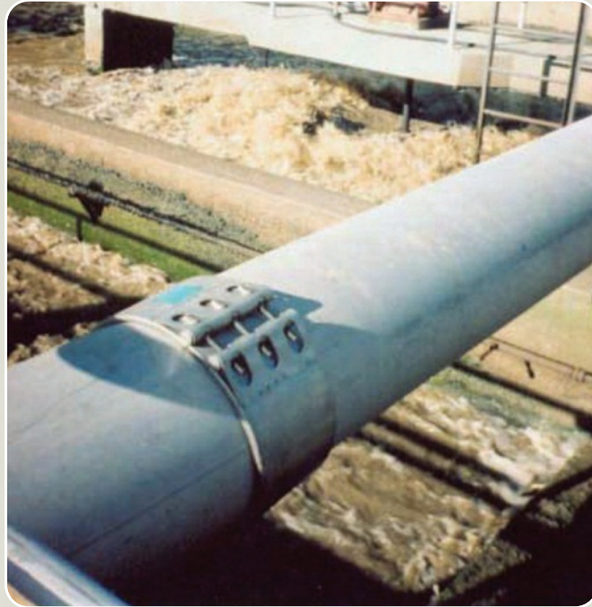
▲ Spain: water purification facilities
