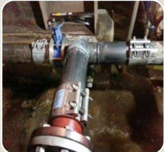
▲ Netherland desalination treatment facilities
